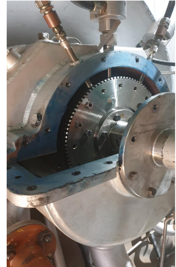
Turbine Non - Drive End
