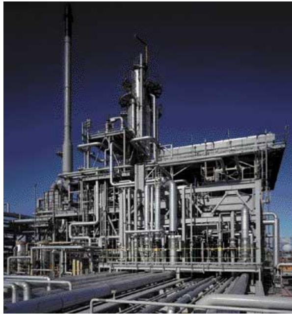
Figure 3: Hydrotreater Unit Grangemouth, UK
