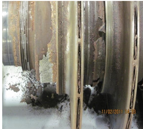
Figure 27: Ammonium Chloride Fouling in a Hydrogen Recycle Compressor
