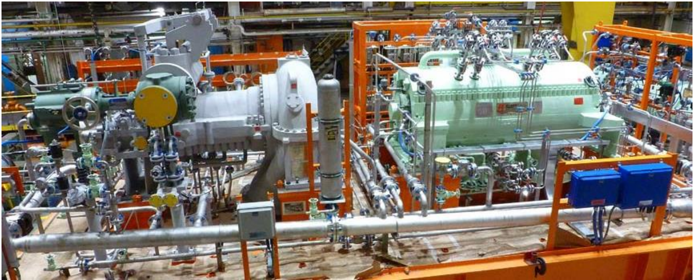
Figure 11: Steam Turbine Driven Wet Gas Coker Compressor
