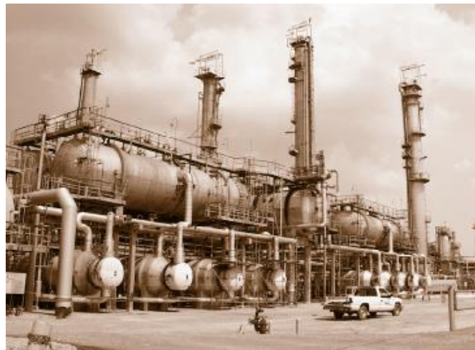
Figure 8: Alkylation Plant (Courtesy of Motiva)
